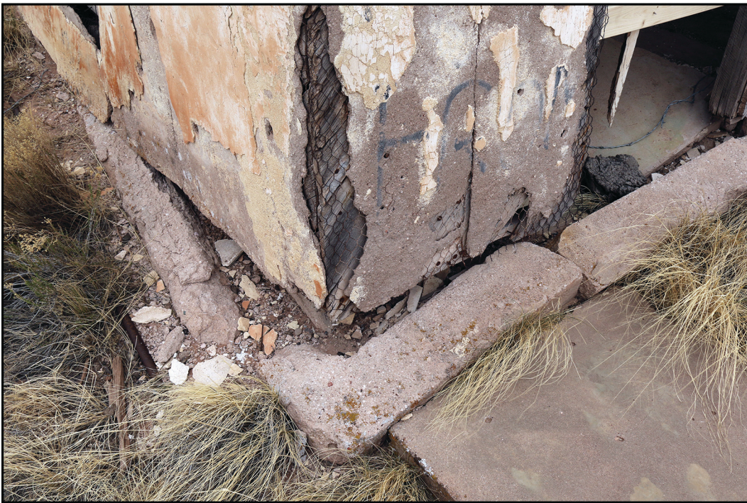
Detail view of the northwest corner, showing the broken and collapsed stem wall.
