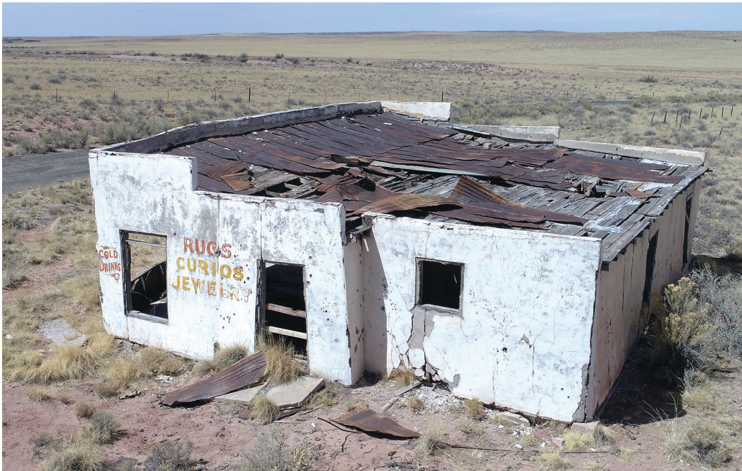
Westward view of overall structure, showing slumped walls and damage to roof.
