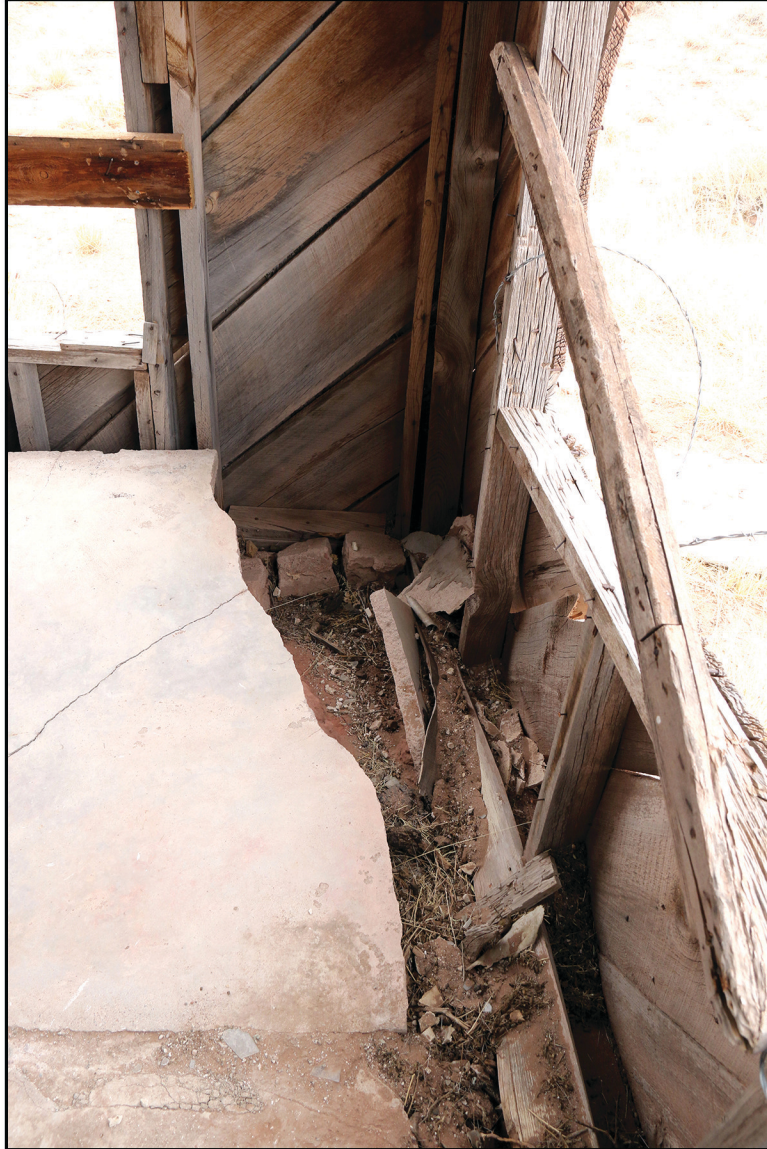
Interior view of the southeast corner, showing the relationship between the slab floor and the walls.
