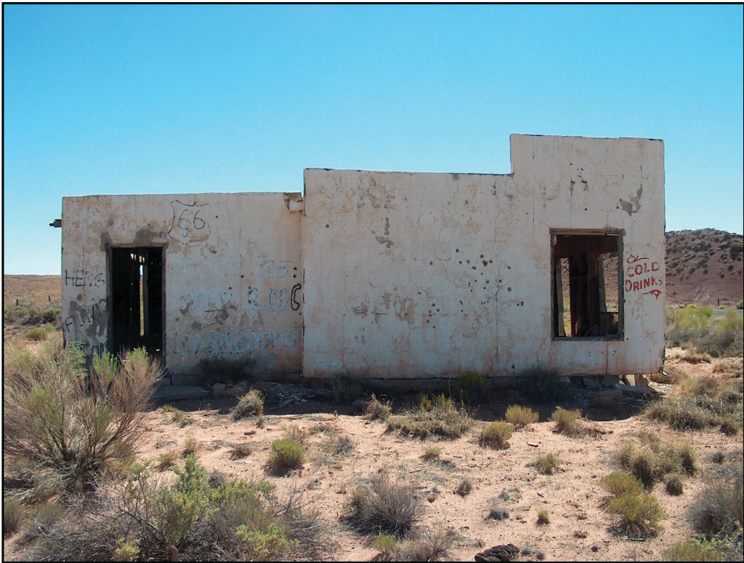
West Wall. Note the void beneath the southwest corner.
