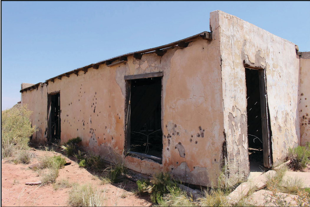
View of the northwest corner and back wall, showing failure of stem wall that once supported the building's exterior walls.
