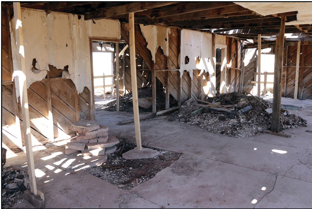
Interior view in present condition looking toward the northeast. Debris has been raked into piles and temporary supports installed to help stabilize the structure.
