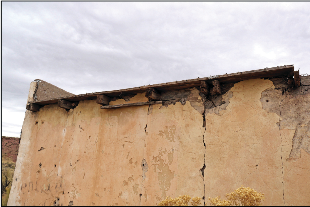
View of the roof's edge along the back wall at the east end of the building.
