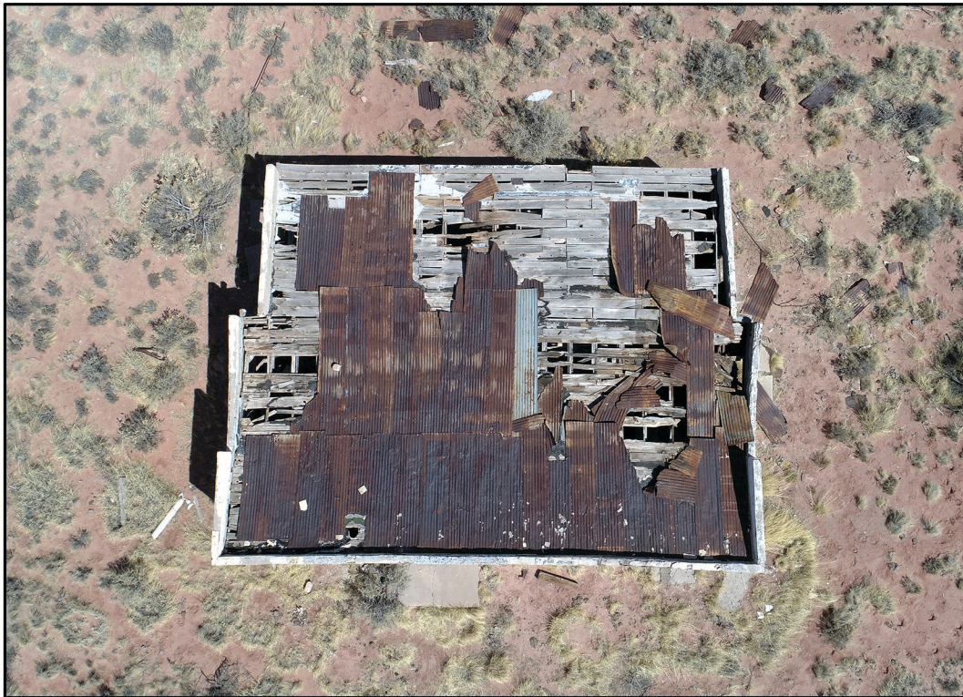
View of the roof from above showing the condition of the sheet metal and the rotted condition of the decking. The building's front is at the bottom of photo.
