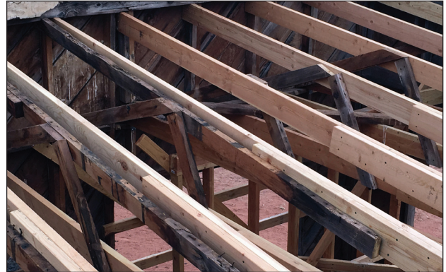
Parts of original rafters attached to new ones, along with use of original diagonal braces.
