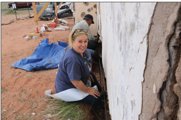
Installing the new sill plate often required workers on both sides of the wall.
