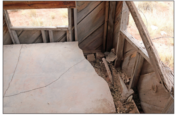
SE corner resting on ground 16" below the floor.
