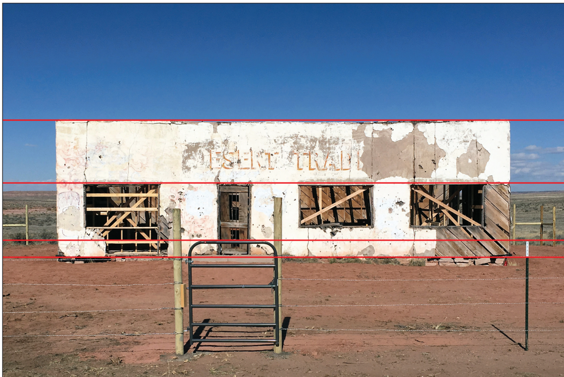
The conclusion of Phase I. The top of the gate is level, as are the red lines, illustrating the relative success of the wall raising.
