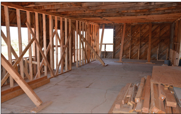
Front room shear wall and added braces. Photo taken after completion of Phase III.
