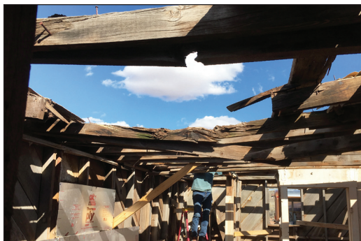
Rotted ceiling in rear room.
