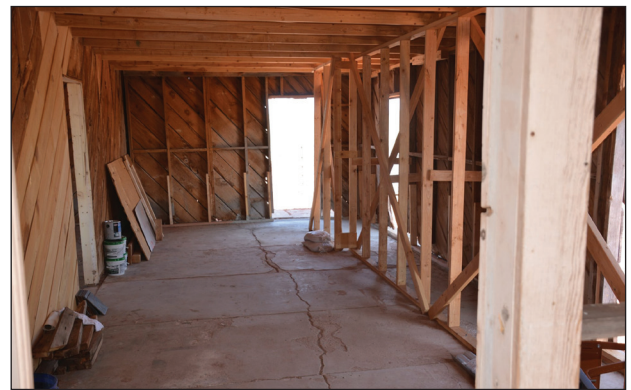
Shear wall in back room (right side of image). Photo taken after completion of Phase III.
