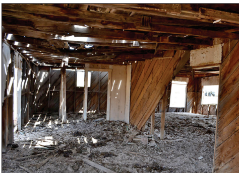
Debris covering the floor.
