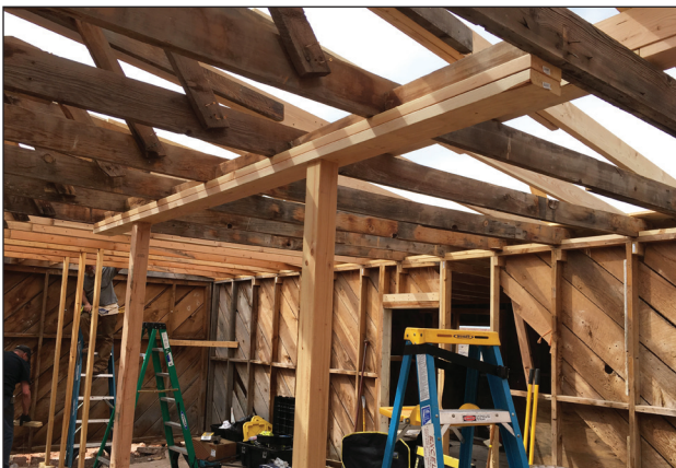
Jack posts were used to raise the sagging original front room joists on plane with the new ones. They were then secured to the stiff-back.
