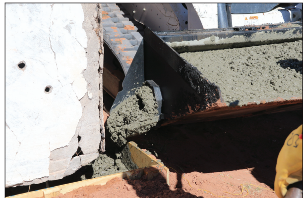
A patent-pending bucket designed and owned by one of the Co-Op members was used to dispense concrete.
