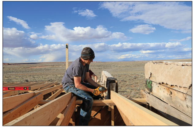
A front room rafter being secured to the main partition wall. View toward the north.
