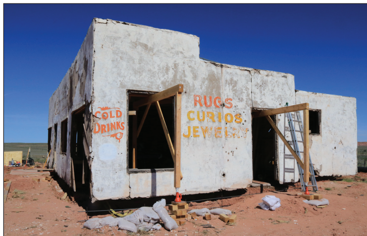
The interior shear walls, along with angled wall supports and beams positioned through window and door openings were used to “levitate” the building so that remaining temporary supports beneath the walls or otherwise obstructing access to the foundation could be removed.
