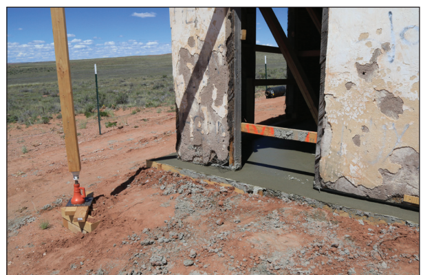
The NW corner of the trading post now rests on solid concrete.
