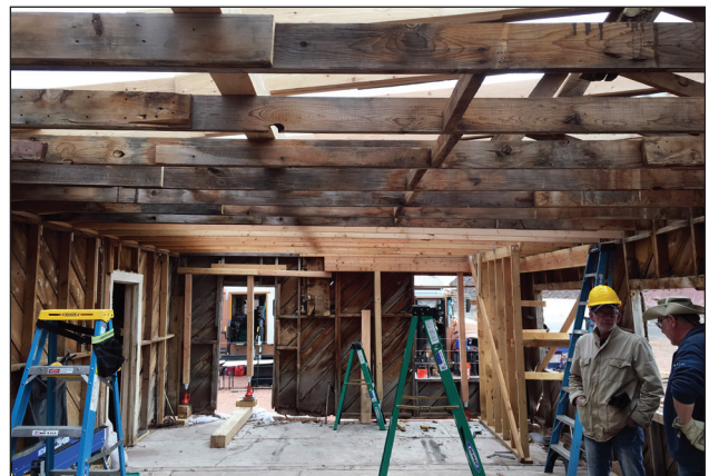
Seven of the original ceiling joists in the middle of the main room were preserved intact. The stiff-back can be seen across the tops of the joists in the upper left portion of the photo.
