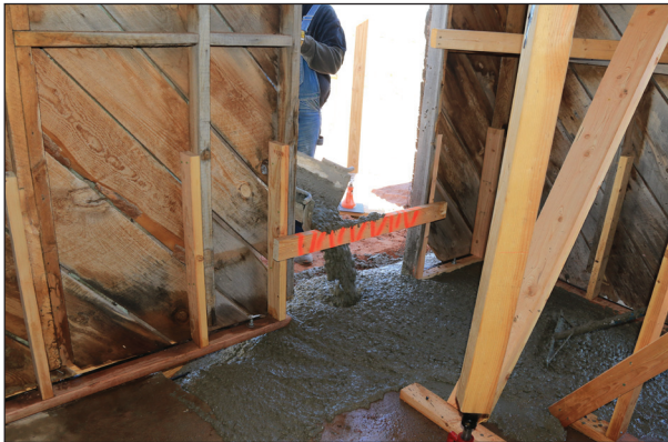
The concrete truck's chute quickly filled large areas where voids in the slab existed.
