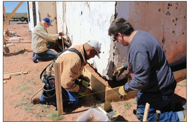
The concrete forms had to be the same height as the slab floor inside the building.
