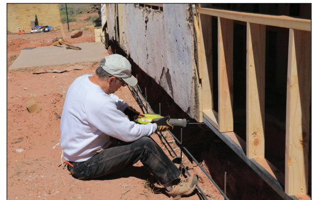
Stucco and the wood sheathing behind it was trimmed to match the bottom of the new sill plate.
