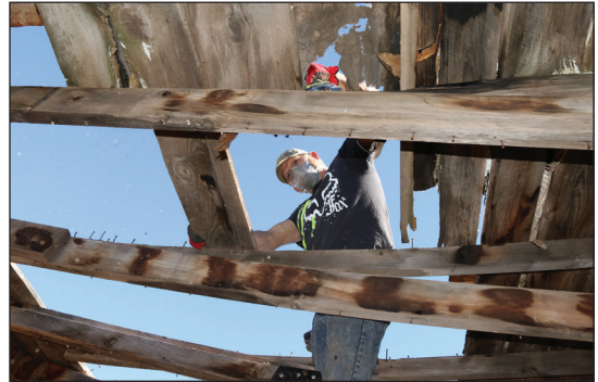
All of the original roof decking had to be removed and replaced.
