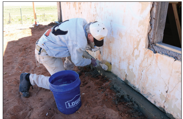
Concrete splatters were cleaned from the stucco immediately after the concrete was poured.
