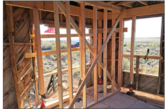
View of the shear wall on the west end of the building's front room.
