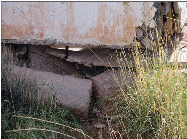
Foundation and sill plate separated from wall. NPS
