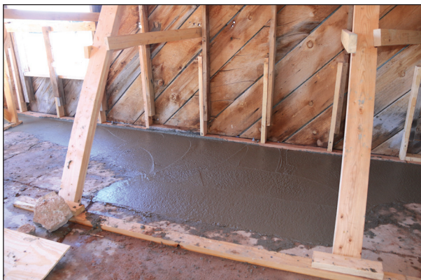
Here the slab and foundation become one. Note the "sistering" of wall studs to the new sill plate.
