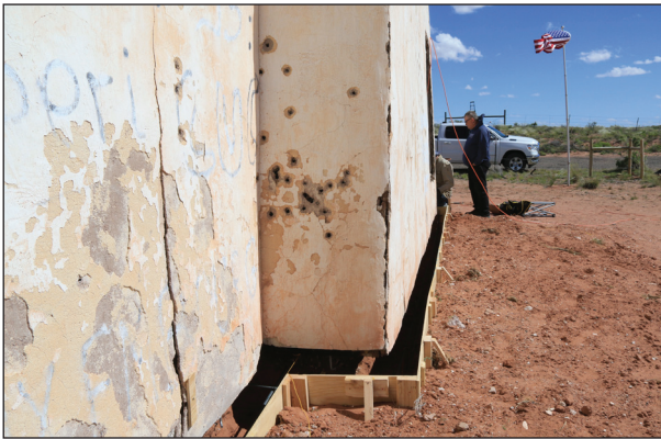
The foundation forms were made of plywood and backfilled with earth prior to pouring the concrete.
