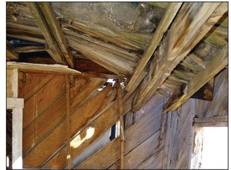
Roof collapse at east end of partition wall. NPS
