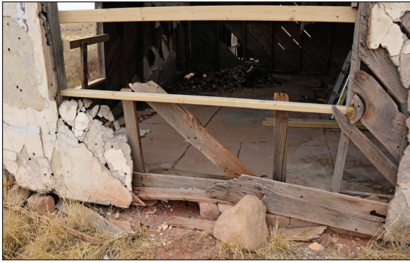
Cattle damage - west front window.
