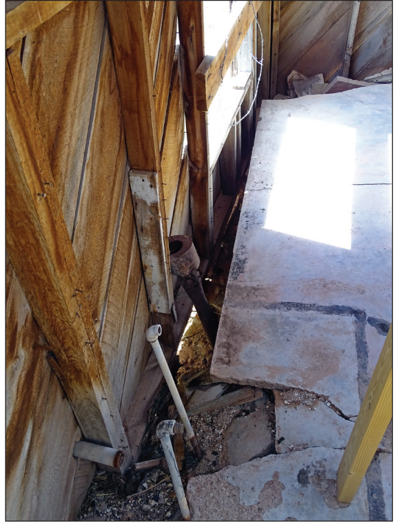
East Wall (view toward front) illustrating fallen wall due to foundation failure. NPS
