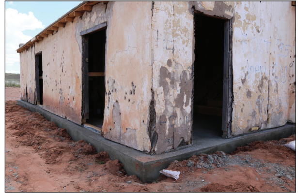
View of the north (rear) and west walls from the NW corner.
