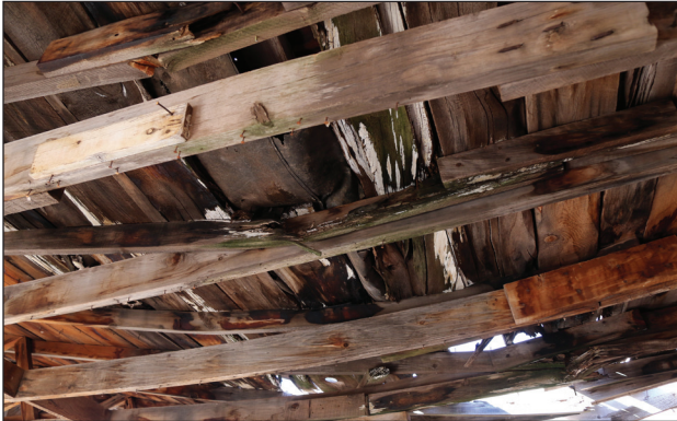
Condition of existing rafters and joists at the east end of the front room.
