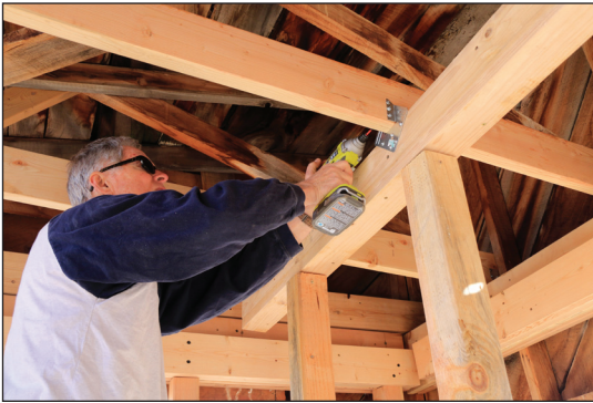
Securing a jack post beam to a replacement ceiling joist on the SE corner of the building.
