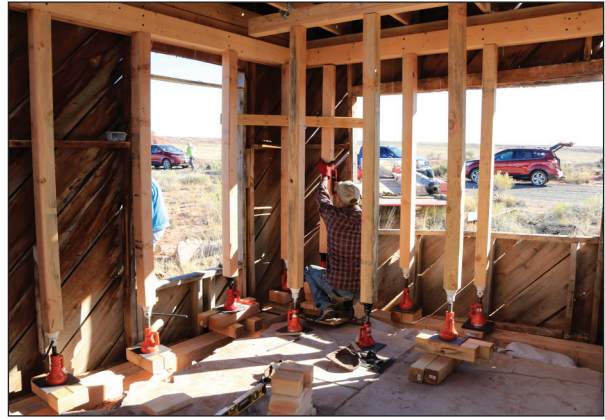
SE corner with double row of jack posts. Note use of timbers and sand bags beneath jacks.
