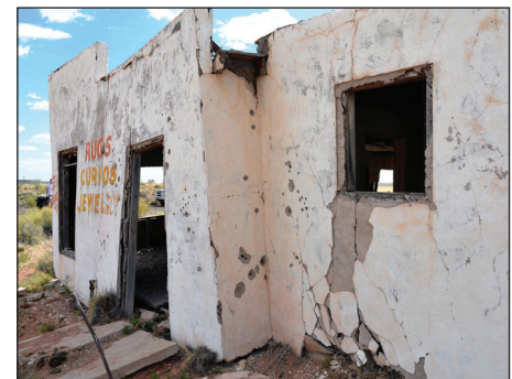
Bottom of wall pushed away from building (near door opening); cattle damage to stucco.
